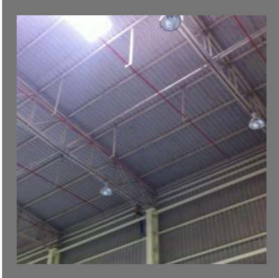
Bird Control Netting
